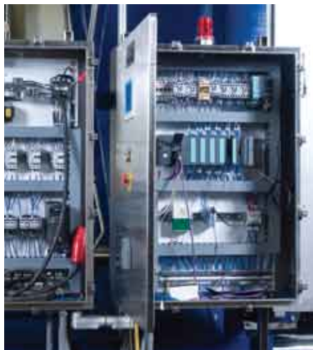
View of inside of the PLC control panel.
